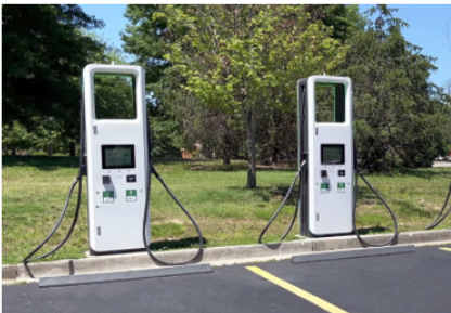
Provide Preferential Parking Spaces for Electric Vehicles
