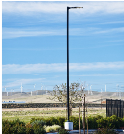
Typical Single-Head Parking Lot Lighting
